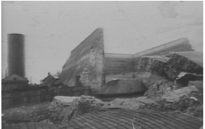
Photo showing the collapsed north wall of the reservoir. The standpipe at left was already being used as part of the town water supply. (Forsyth County Public Library Photo Collection)
